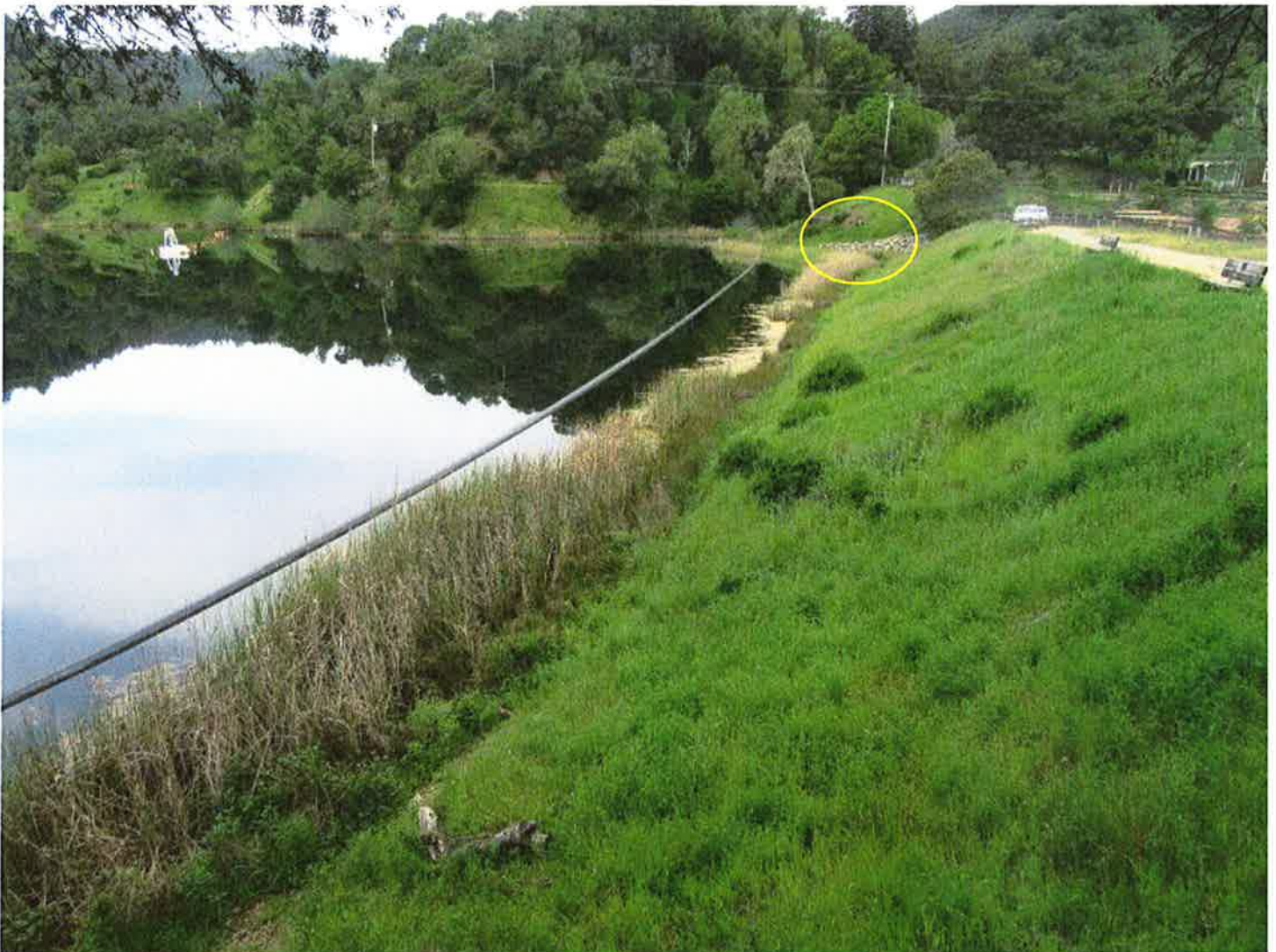
The upstream face as viewed from the right abutment. Tule and cattails along the upstream face waterline should be cleared before the next periodic inspection. The location of the spillway entrance is circled.
