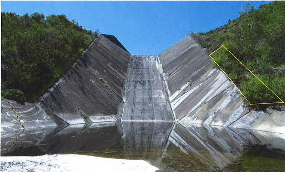
The spillway and flip bucket looking in the upstream direction. Large bushes along the lower left spillway wall should probably be trimmed back a bit to prevent possible root damage.
