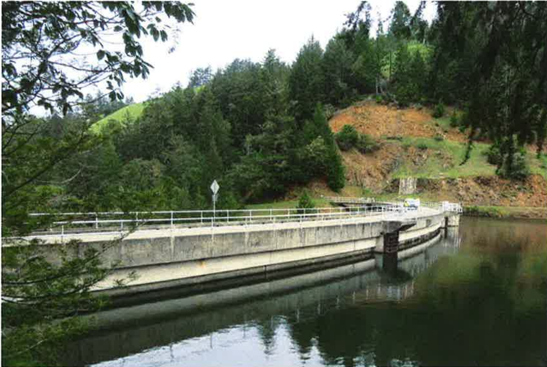
The upstream face as viewed from the left abutment. The reservoir water surface elevation is 0.1 feet above the spillway crest.
