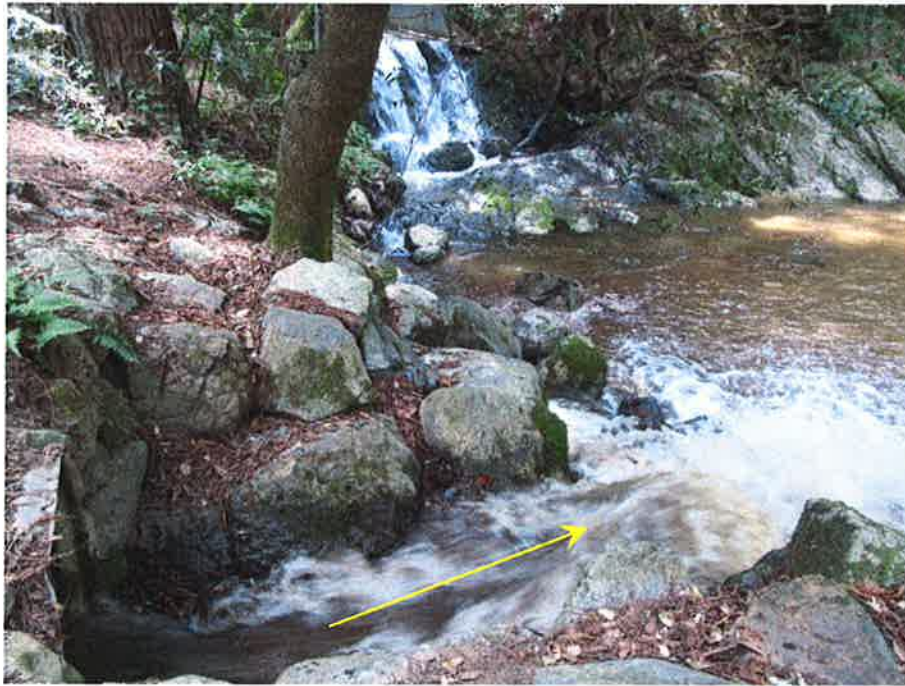
Flow from the full head outlet test of the 16-inch upstream control and 10-inch downstream control is visible in the lower half of the photograph. Flow from the spillway outfall can be seen in the top center of the photograph.
