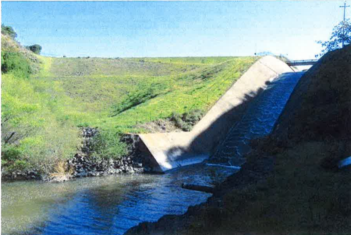
The downstream face, spillway outflow channel, and stilling basin. The outlet discharges into the stilling basin just upstream of the drain pipe visible in the bottom center of the photograph.
