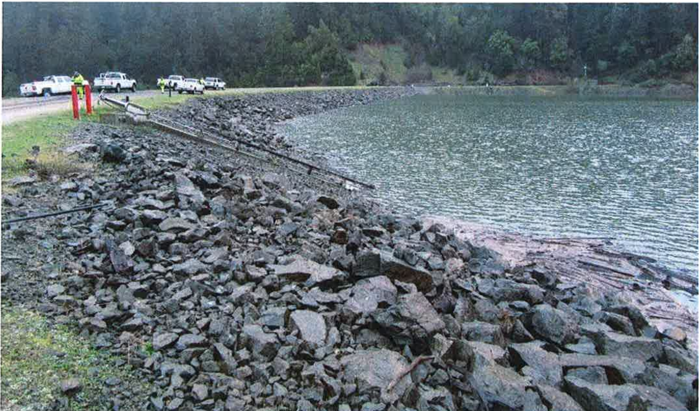
The upstream face as viewed from the left abutment. The large boulder rock riprap upstream face protection remains in good condition.
