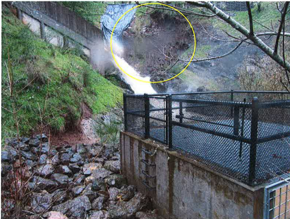
A small rock fall has occurred within the lower left abutment just below the concrete spillway channel outfall (circled); the rock fall did no damage to the lower spillway channel.
