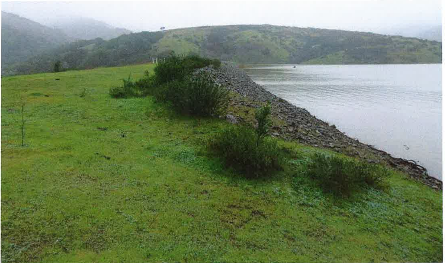
The upstream face of the embankment as viewed from the spillway entrance.
