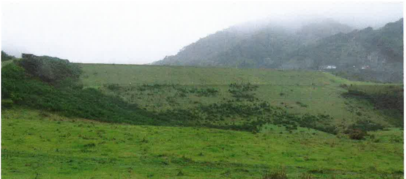
The downstream face of the embankment as viewed from the alternative access road.
