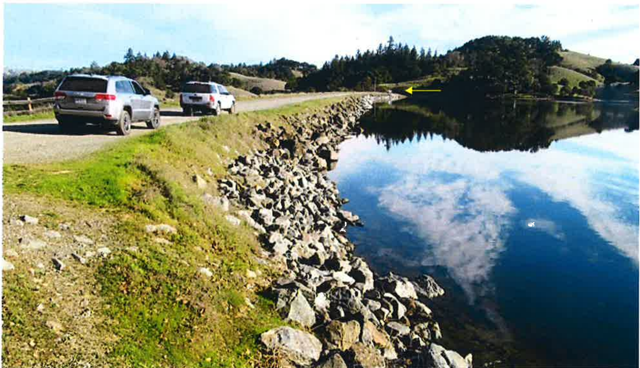
Another view of the upstream face, this time looking towards the spillway entrance.
