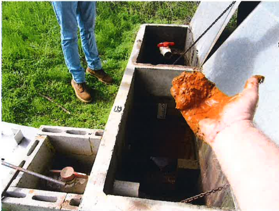
The seepage collection box has a significant accumulation of sediment. I asked Ms. Croy to ascertain the source of the sediment, and recommended running a sieve analysis to better identify the materials collected. The concern is that the sediment may be the result of internal erosion. I also asked that the box be well cleaned to facilitate monitoring for additional sediment accumulation.
