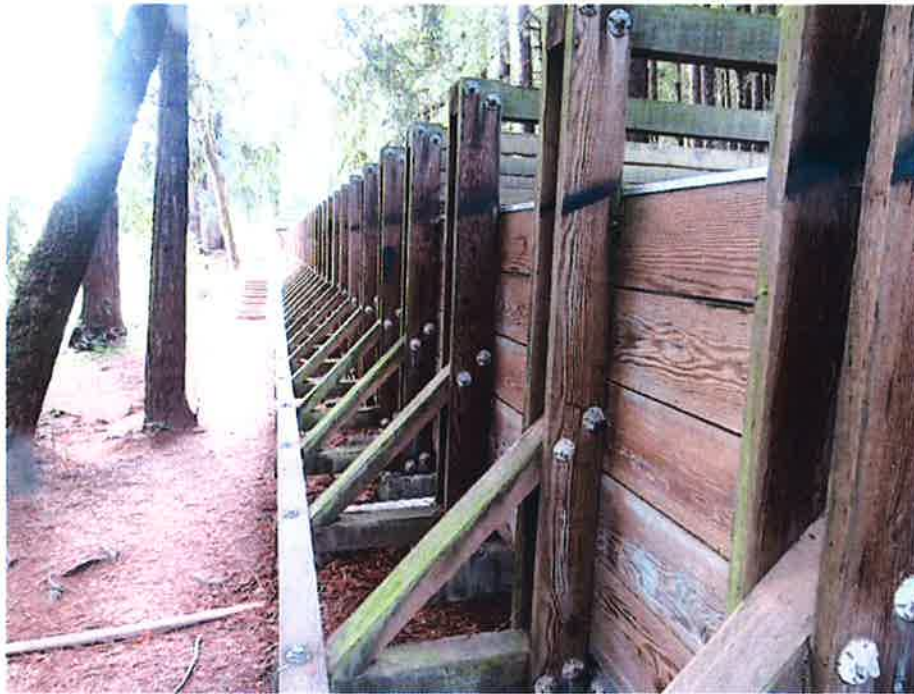
Pressure treated timbers supporting the flume appear to be in good condition, as does the stainless-steel flume sheathing, the under flume supports, and flume foundation connections.
