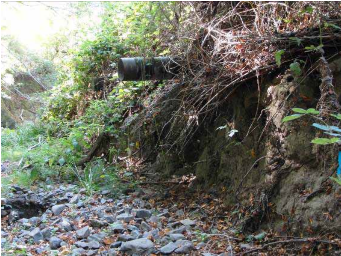
Figure 20. Lagunitas Booster Station streambank stabilization site, on San Geronimo Creek (eroded streambank and discharge pipe), looking upstream (top) and downstream.
