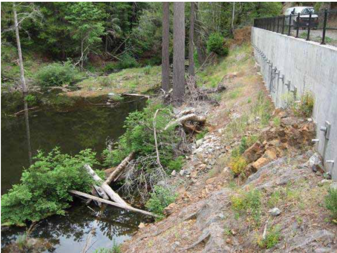
Figure 21. Below Peters Dam streambank stabilization site; top view looking upstream towards Peters Dam, bottom view looking downstream.
