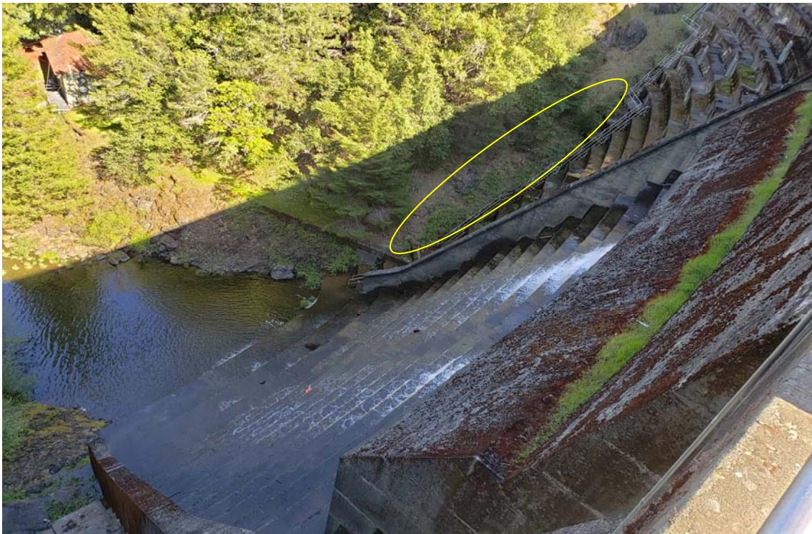
Photo 3: View of the downstream face as seen from the left abutment. Minor vegetation in the right groin (circled) requires removal.
