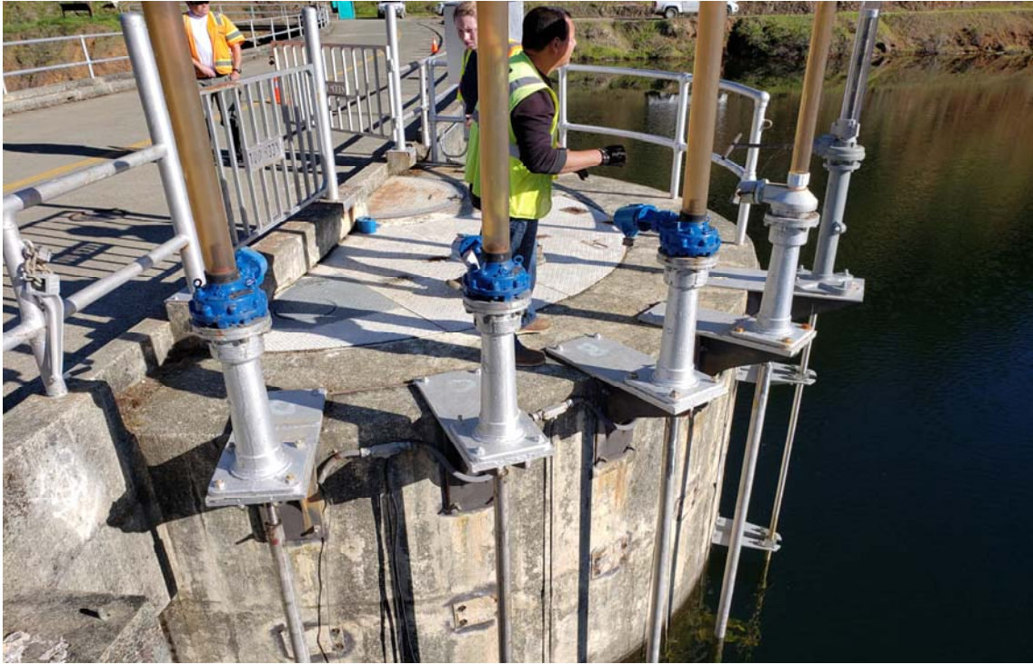
Photo 2: View of the recently replaced valve stems for the upstream slide gates.
