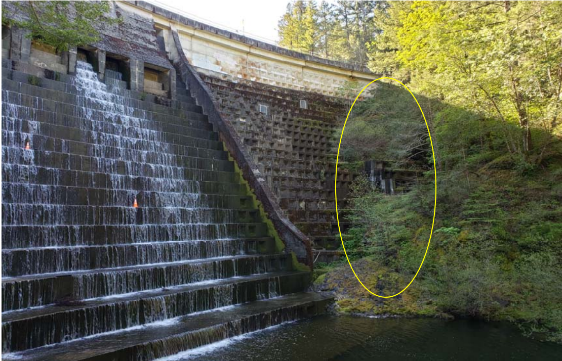
Photo 4: View of the downstream face looking towards the left abutment. Vegetation in the left groin (circled) requires removal.
