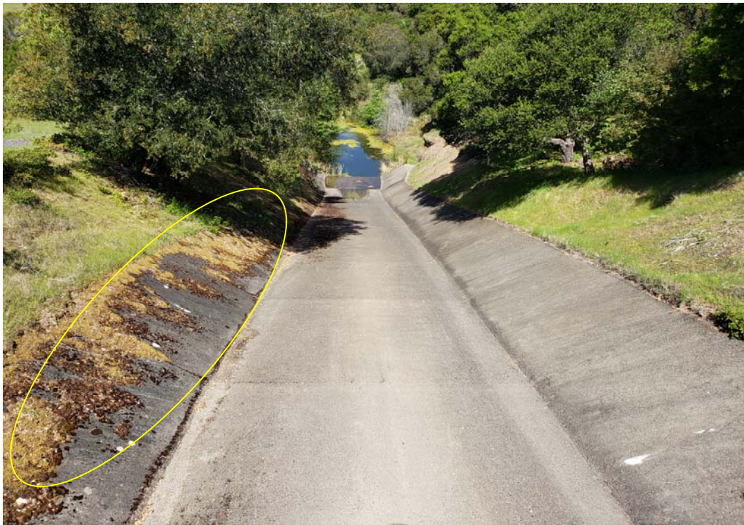
Photo 4: Vegetation growing in the spillway joints needs to be removed.
