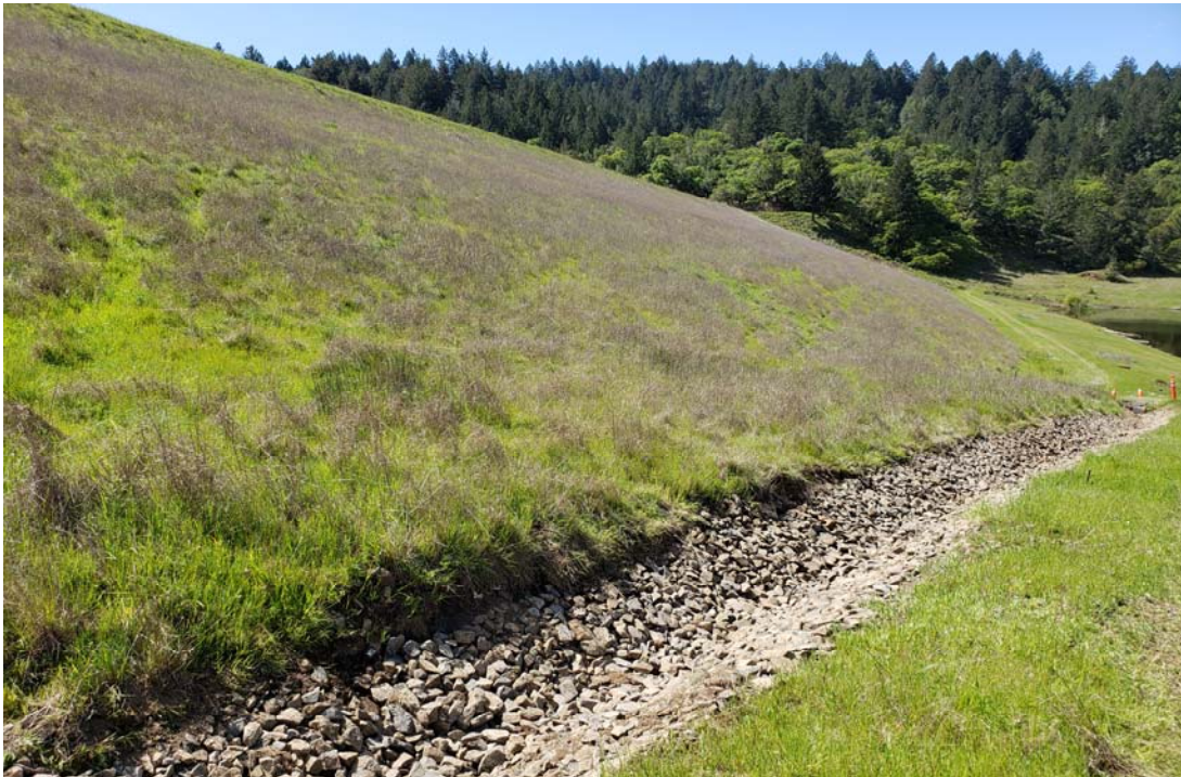
Photo 2: View of the downstream face and seen from the right abutment, and the replaced rock in the drainage ditch.
