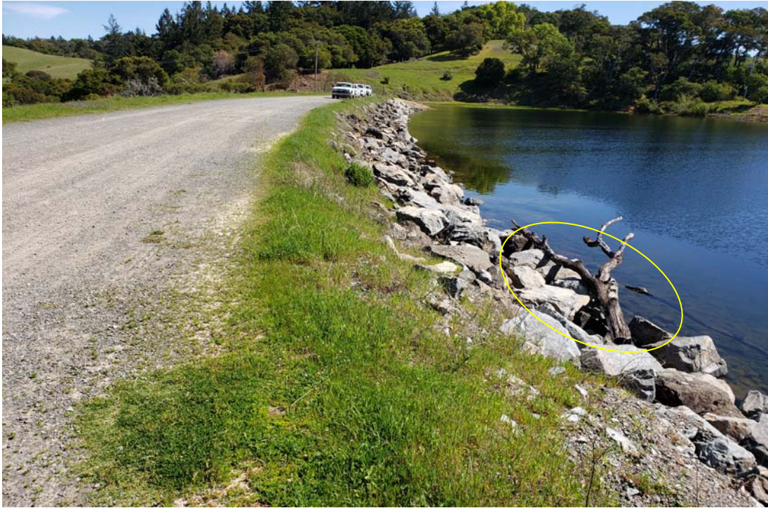
Photo 1: View of the upstream face looking toward the right abutment and spillway. The circled debris needs to be removed.
