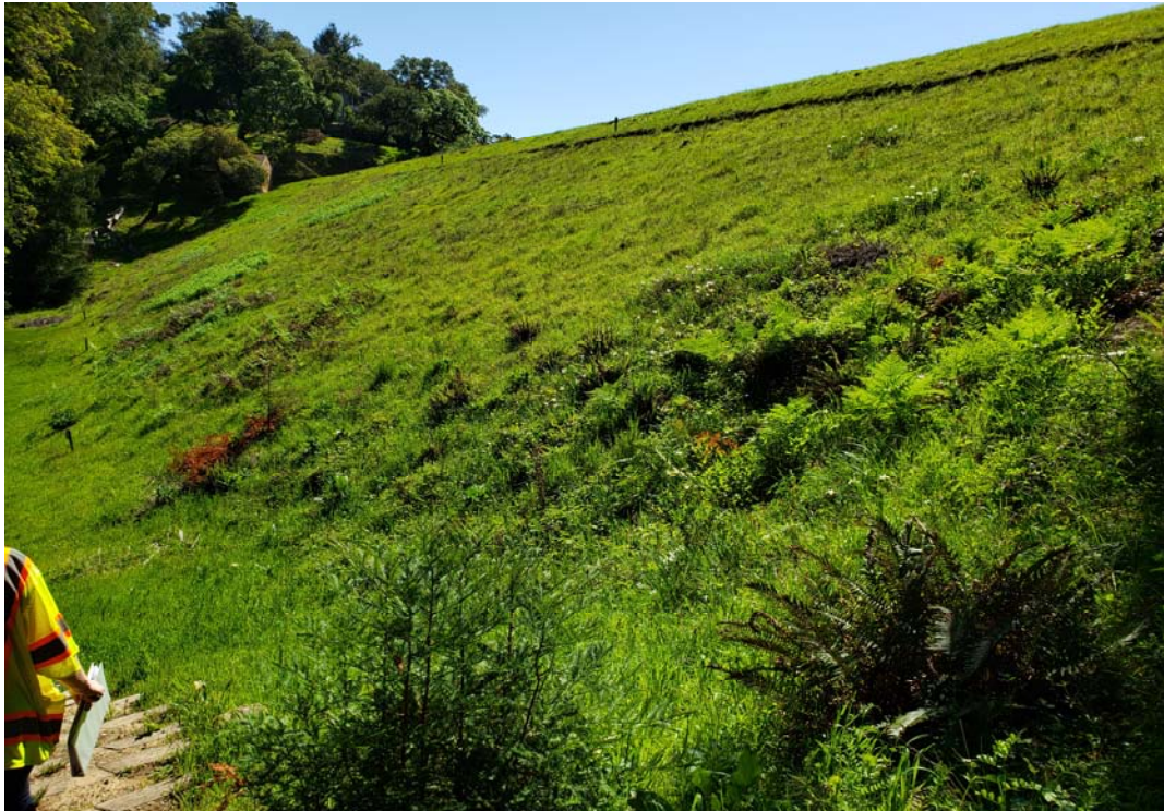
Photo 2: View of the downstream face as seen from the toe. Patches of dense vegetation need to be removed.
