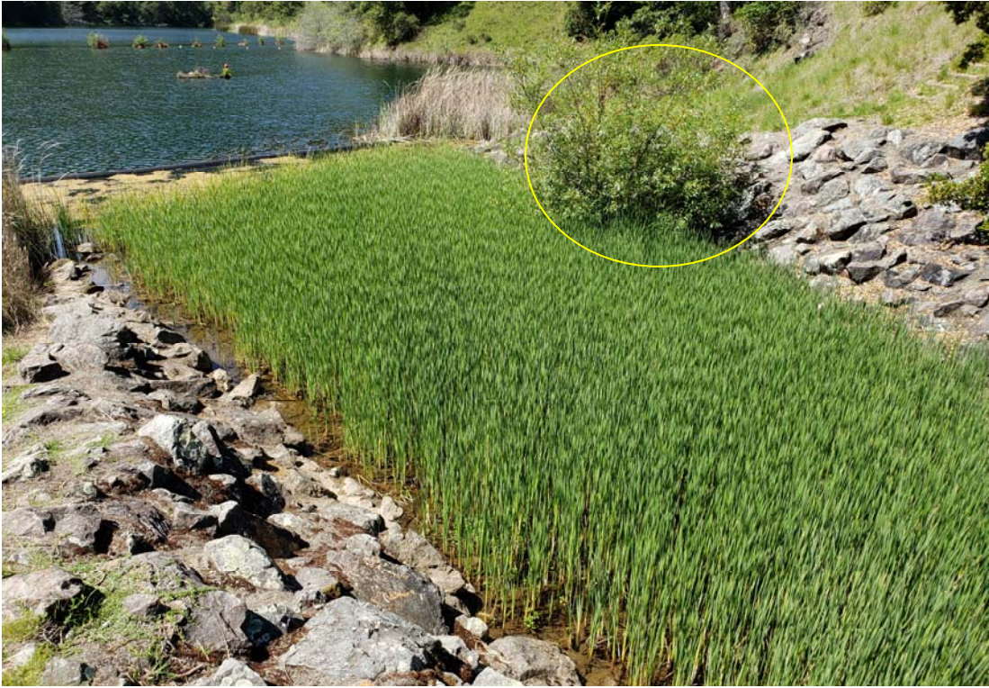
Photo 3: Tules and the circled tree in the spillway approach need to be removed.
