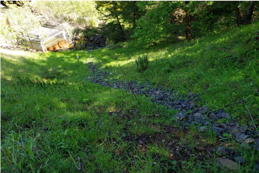
Photo 4: Additional rock was placed in the groins of the lower portion of the downstream face.
