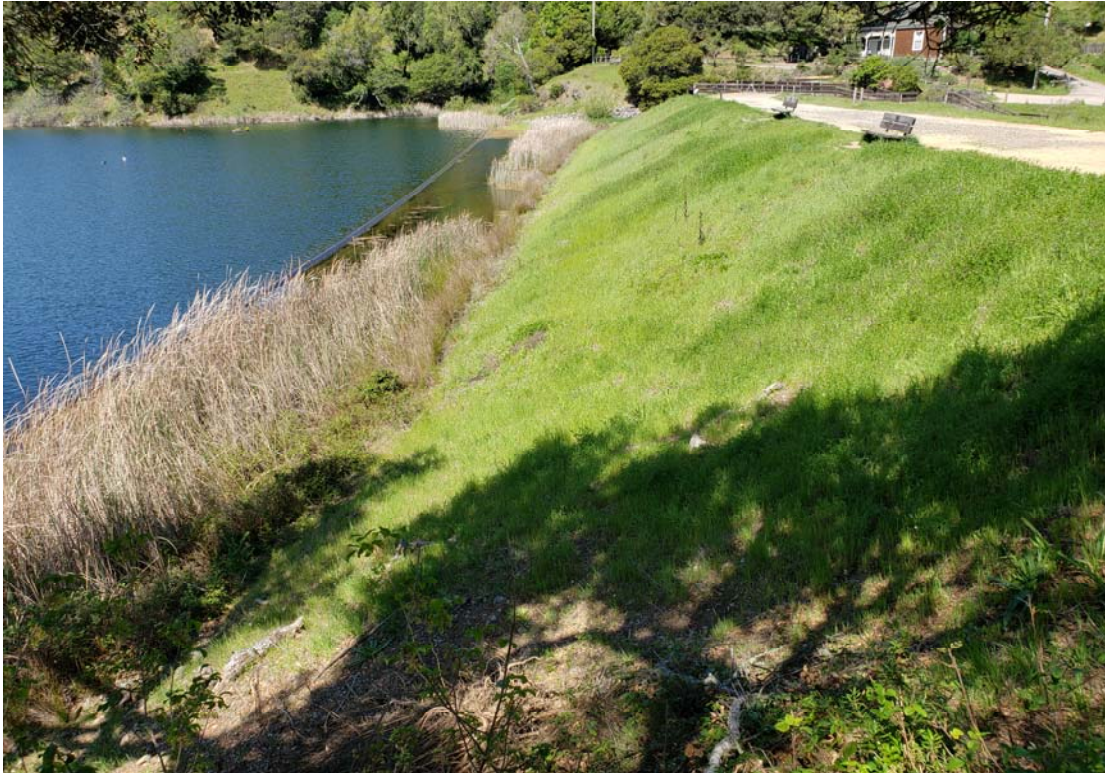
Photo 2: View of the upstream face as seen from the right abutment. Tules along the waterline (circled) need to be removed.
